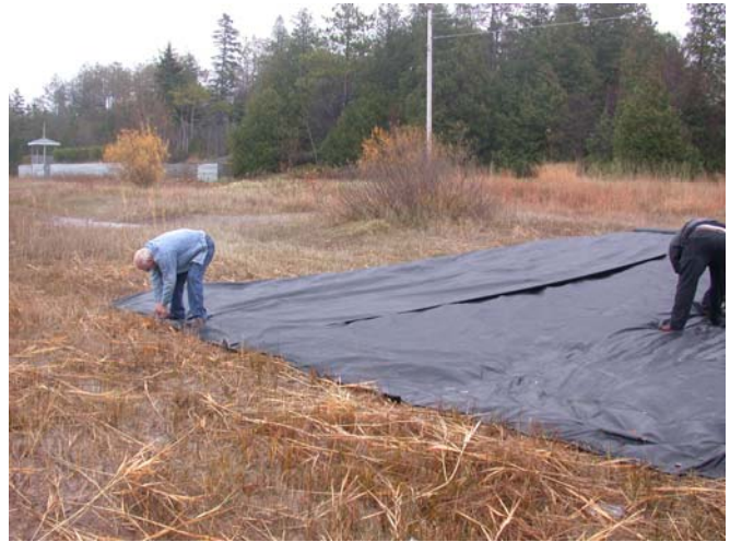
Installation of black geotextile blanket over a freshly cut area. Blanket was left in place for several months with mixed results.
